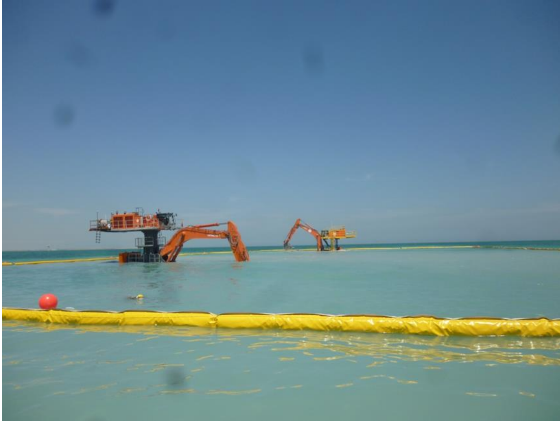
Figure 3. A view of the deployed silt curtain around the trenching site in Abu Ali
